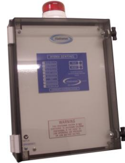
Electrical Control Panel
